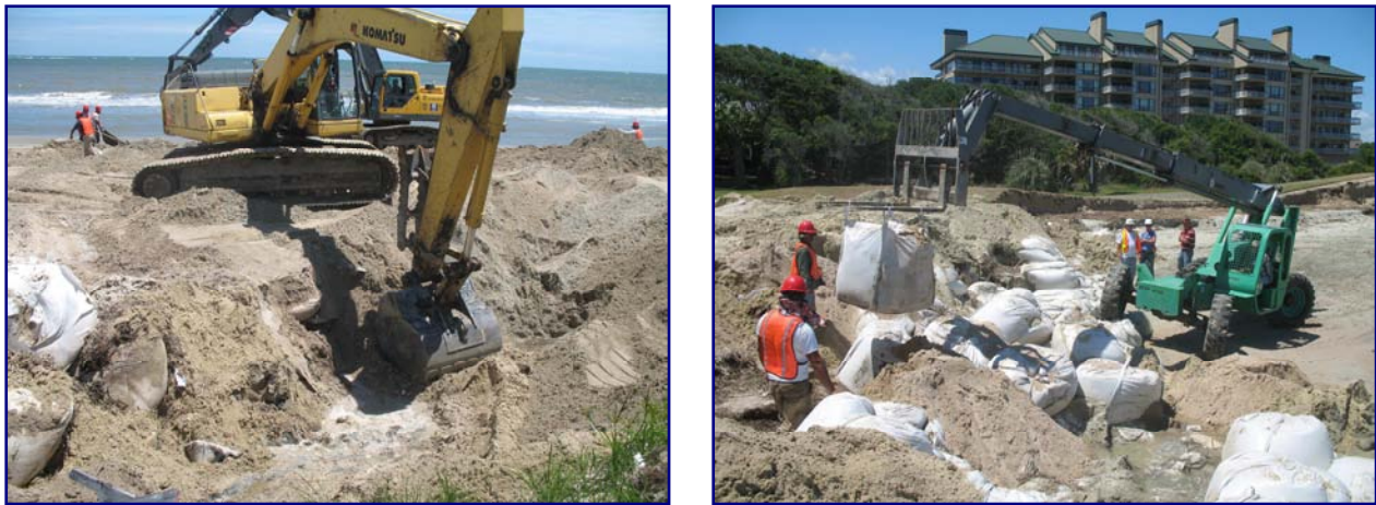
FIGURE 1.7. Contractor, Dirt Cheap Inc, removing sandbags prior to nourishment. In the left image, a track hoe digs to remove buried small and large bags. In the right image, a long-reach forklift removes accessible bags. Material was dumped from the bags and inspected for compatibility. Unacceptable material was removed from the beach by truck. [Photos by S. Traynum]
