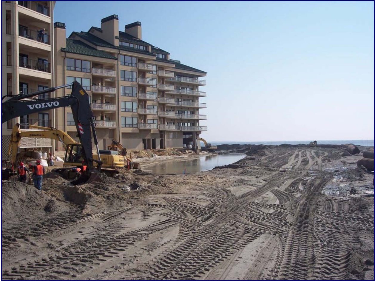
FIGURE 1.8. A temporary berm was built by Weeks Marine to protect buildings and the work area while Dirt Cheap Inc. removed remaining sandbags. Once all bags were removed, the area was re-pumped to fill in the remaining berm. [Photo by S. Traynum]
