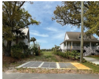
Check valves on marsh outfall
