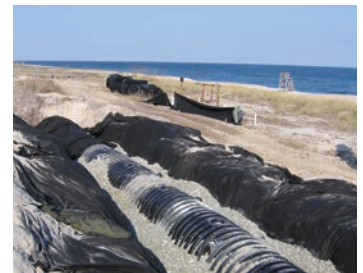
Dune infiltration system
