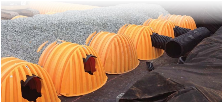
Figure 10 – Infiltration chambers being installed on a project site (photo credit to ADS StormTech).
