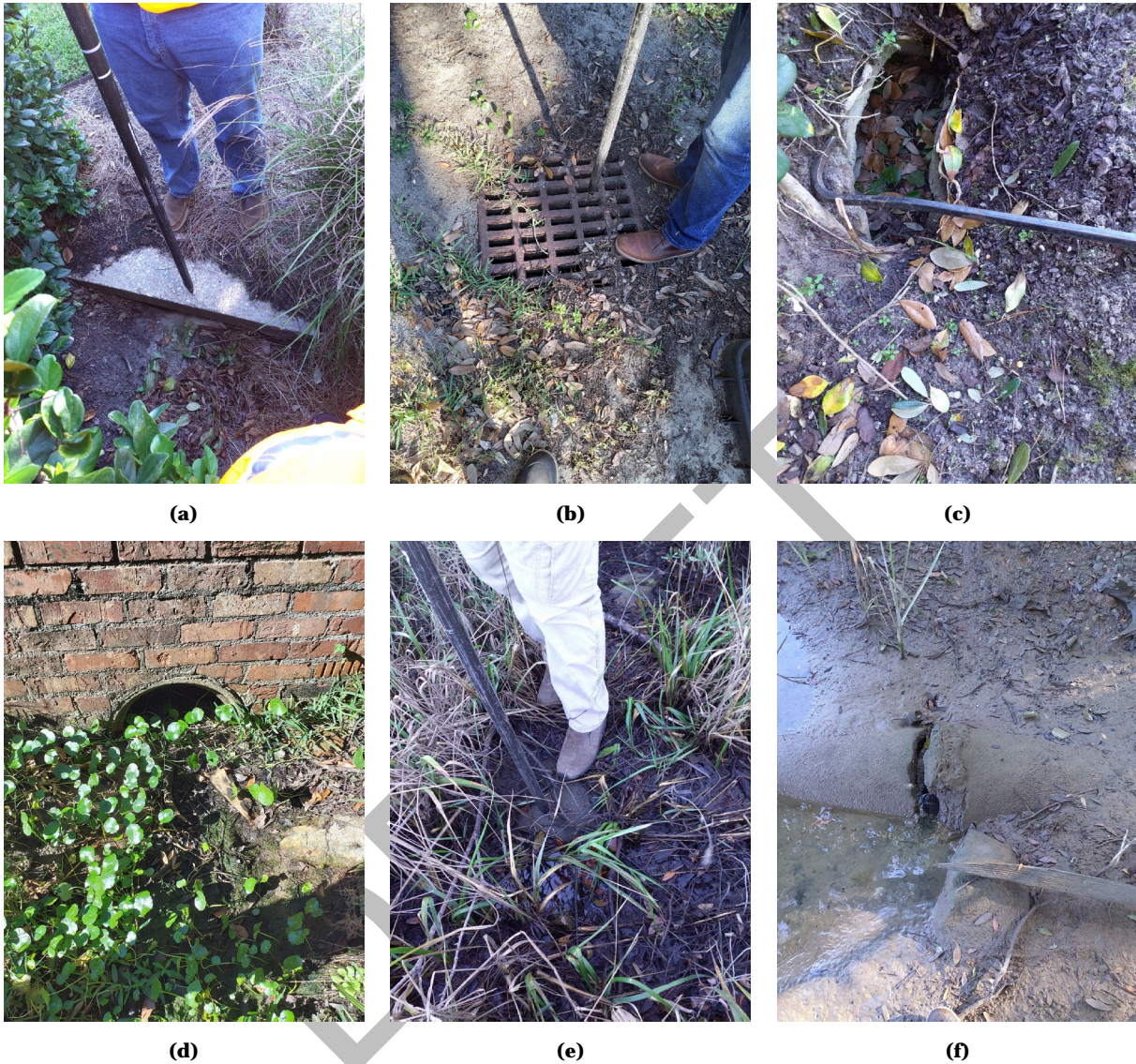
Figure 7 – Examples of visual existing conditions assessments documenting general maintenance deficiencies for: (a) silted inlet; (b) inlet with debris build up; (c) stormwater pipes which have separated; (d) stormwater pipe filled with sediment; (e) buried outfall pipe; and (f) degrading disjointed outfall pipe.
